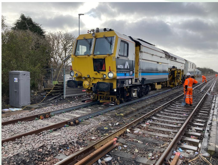
The team working to install new tracks on the line leading into Ashington Station.
